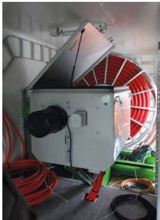
Inside of the container at time of installation
