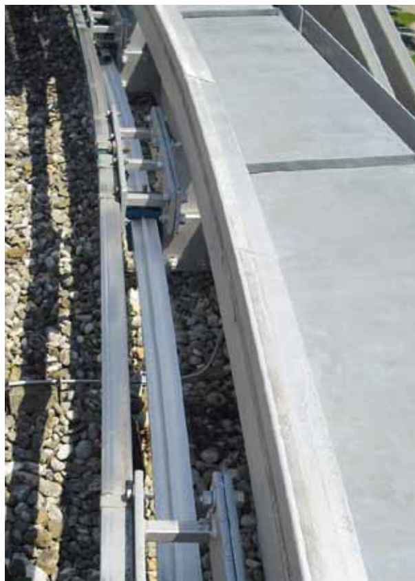
SACL system application
